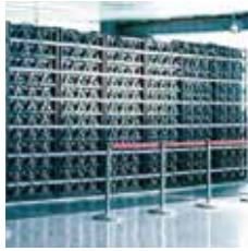
Energy storage system
